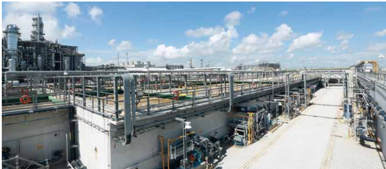
Waste Water Treatment Plant (WWTP) at the Asia Industrial Estate
