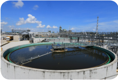
Waste Water Treatment Plant (WWTP) at the Asia Industrial Estate
